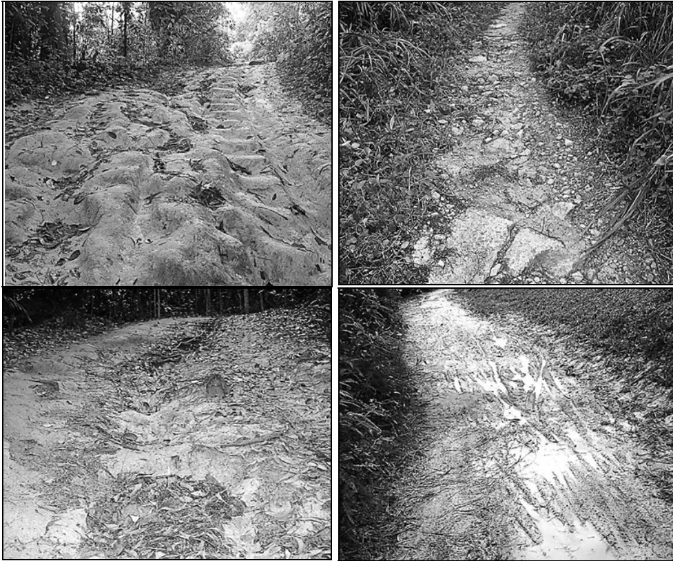
Fig. 11. Surface degradation along trails
